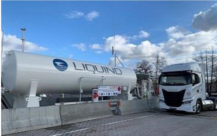
Photo (© LIQUIND): LIQUIND 24/7 LNG filling station in Strullendorf, Bavaria
